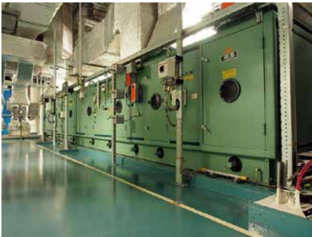
Figure 1. Physical pipelines. An HVAC air handling system for a large data center. Photo: Alf van Beem.
